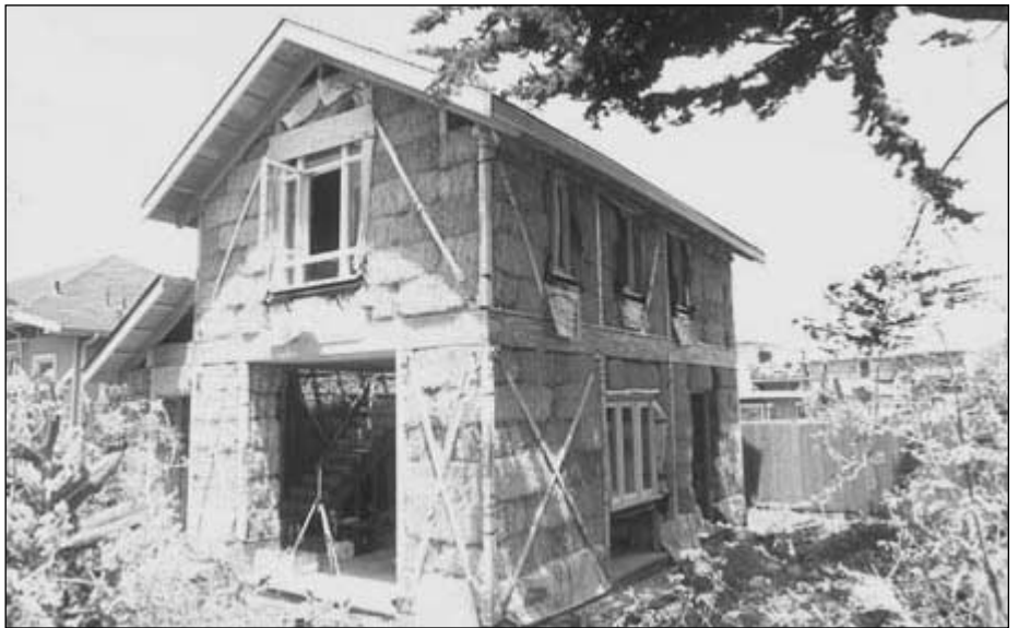
A straw bale home under construction in Berkeley. See the finished look on p. 3.
