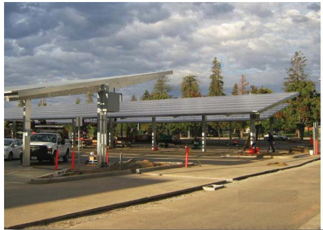
Solar-covered parking lot
